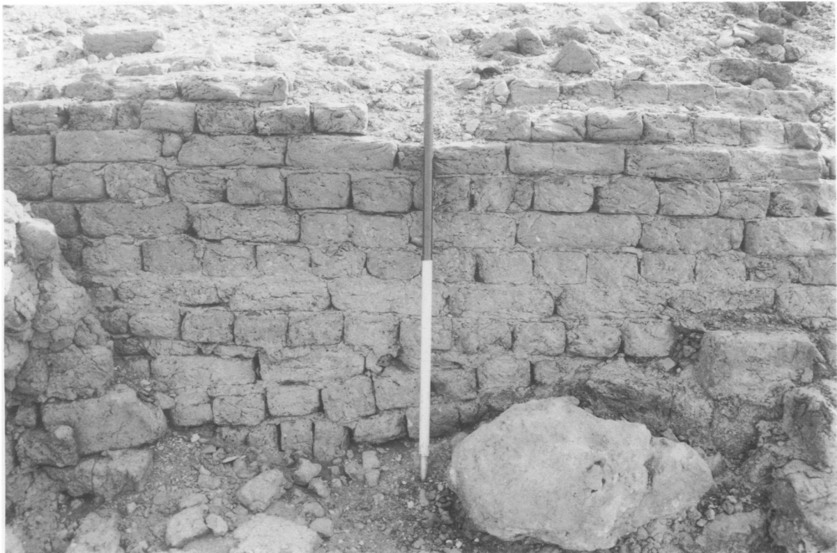
2. Wall at southern end of enclosure, showing foundation courses on natural rock
